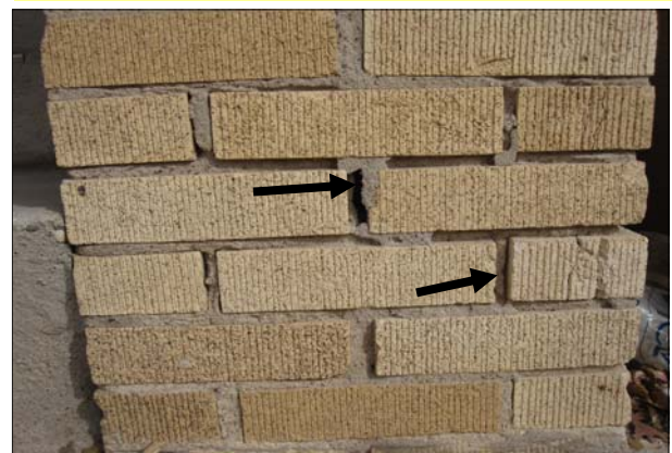
Gaps between bricks and mortar near alley entrance at bottom of steps is one example.
